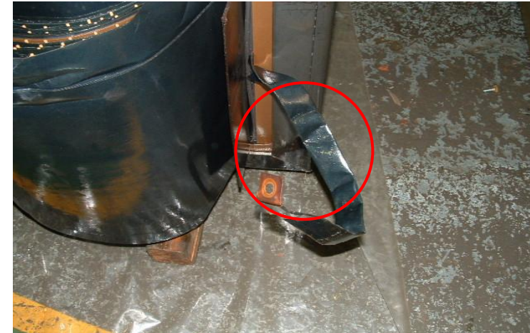
Loose internal earth strip
