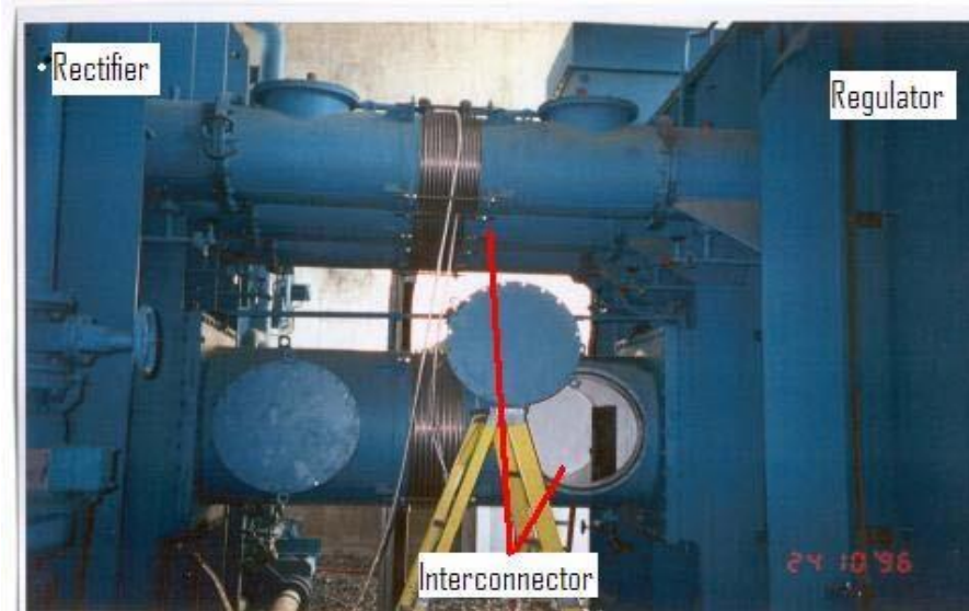
Figure 14 Interconnection system for the Rectifier and Regulator Transformers.
