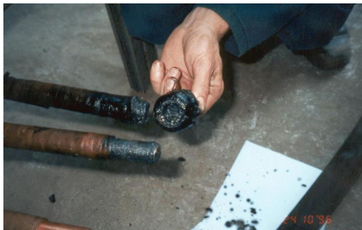
Figure 15(B) Burnt (overheated) connections
