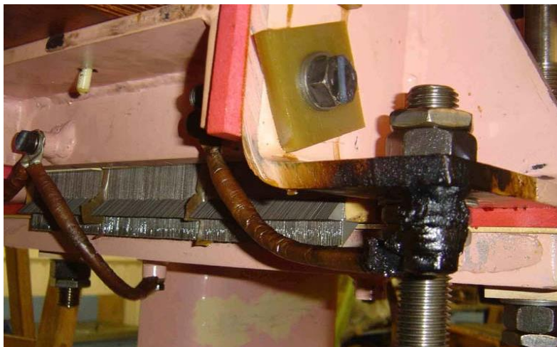
Figure 31: Termination for potential connection became a hot spot due to circulating current
