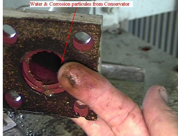
Figure 12-Contaminated Oil (Conservator pipe)
