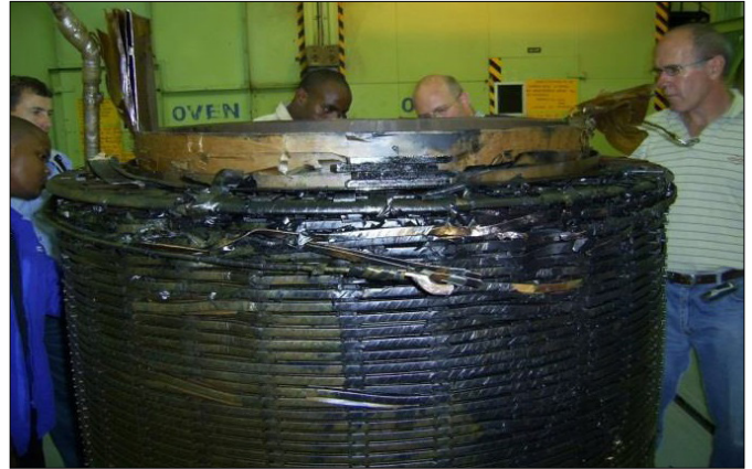
Figure 8: Damage to the HV winding
