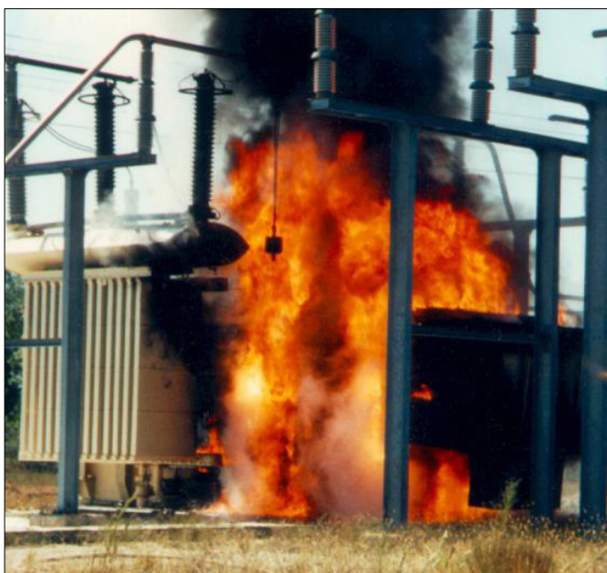
Figure 3: Catastrophic transformer failure
